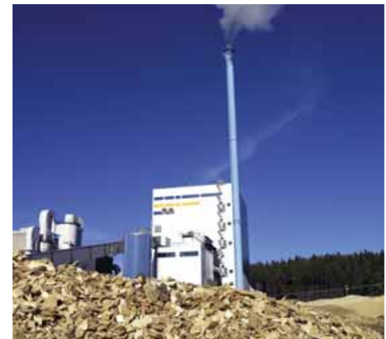
▲ The Våxjö Energy Company's combined heat and power plant at Sandvik. Output: 66 MWh, 36 MWe
